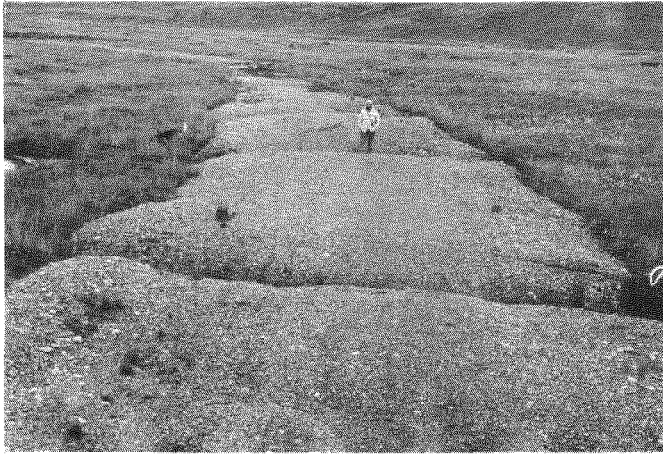
Fig. 5. Roadway destroyed by thawing of ice-wedge tops at Umiat, Alaska. Gravel fill was not thick enough to replace insulating effect of the organic mat which it destroyed (photo by Gordon W. Greene)
